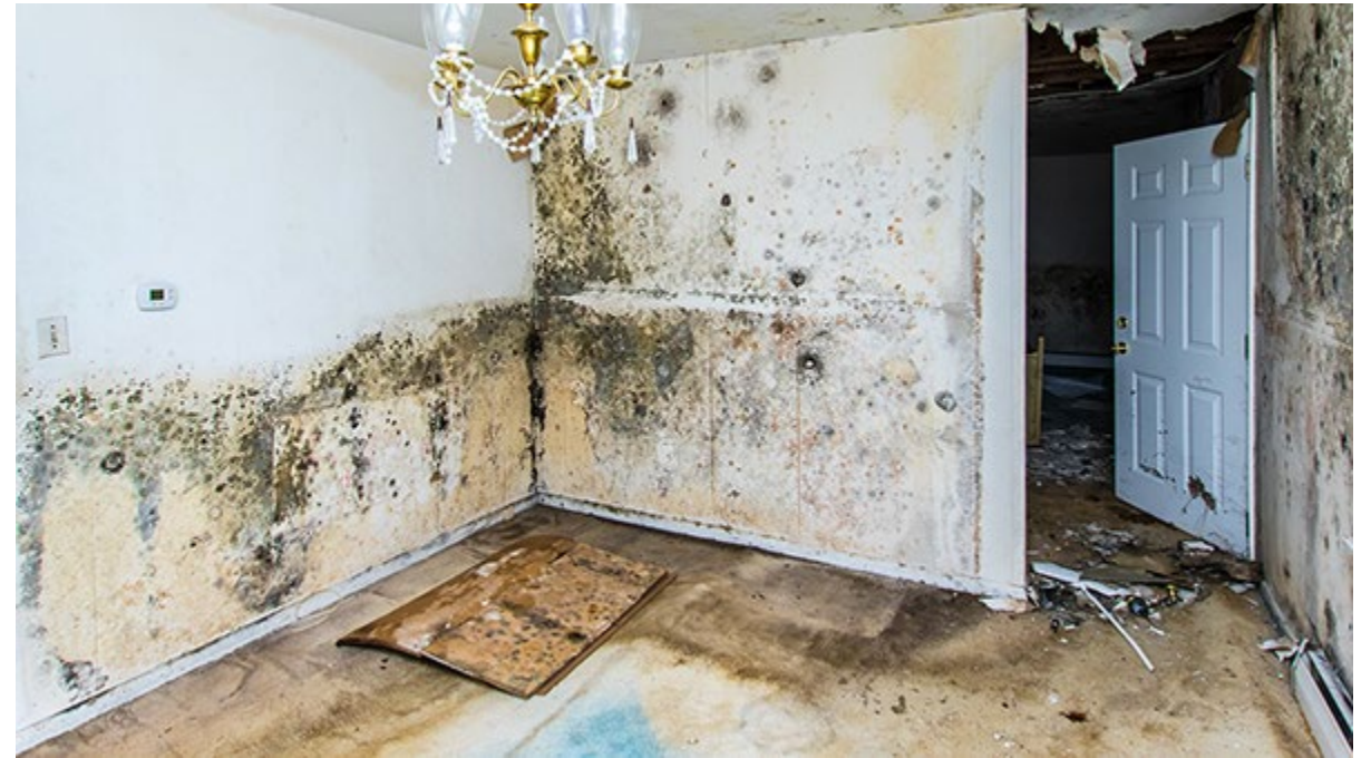
Mold Damage in flooded house, CDC
